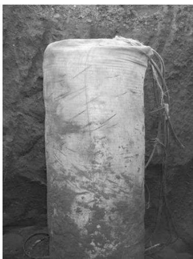
Figure 10. View of the exhumed top portion of the encased column.
