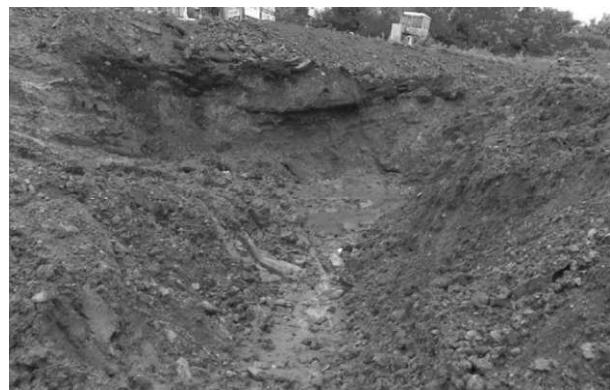
Figure3. The local weakening of the subsoil together with the asphalt overlay and water road filtration.
