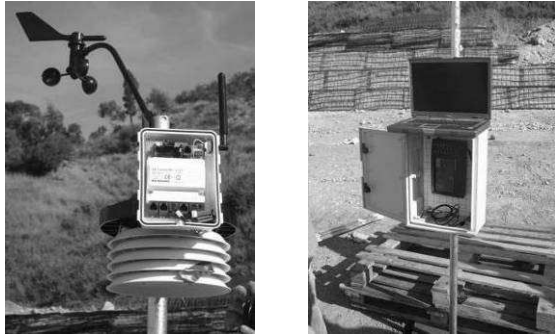
Figure 5. External Weather Station.
