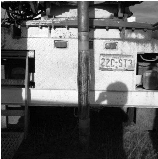
Figure 1. A boring is being drilled prior to the beginning of pressuremeter testing (Courtesy of Kleinfelder Austin Office, 2006)
