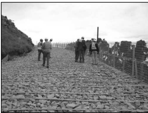
Figure 10. Langeni –galvanized steel reinforcing strips
