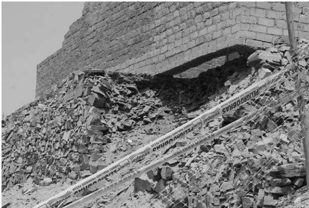
Figure 5. Failure on continuous footing supported on “Pircas”
