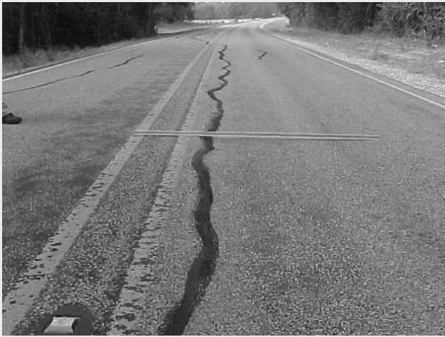
Fig. 3-4 Typical longitudinal crack developed on pavements over expansive clays (Zornberg et al 2009).
