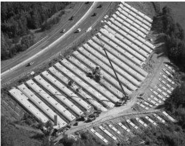
Figure 4. Actual view of the site at motorway A2 from Vienna to Graz.
