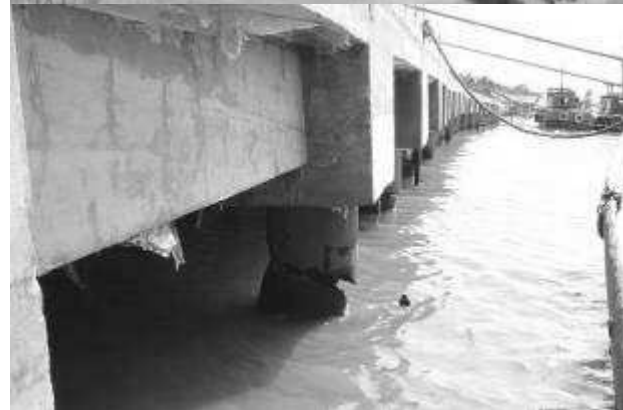
Figure 12. Landslide of riverbank followed by collapse of the structure consists along the riverbank of Barito river.
