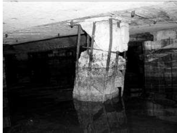
Figure 9. Reinforced concrete piles of the quay after significant physical wear.
