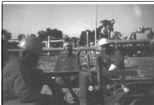
Figure 5: Set-up of the Plate Load equipment for settlement recording versus elapsed time at project site.
