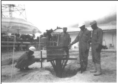
Figure 4: Set-up of the Plate Load Test equipment at the Ogboinbiri Flow station, Niger Delta sub-region, Nigeria.
