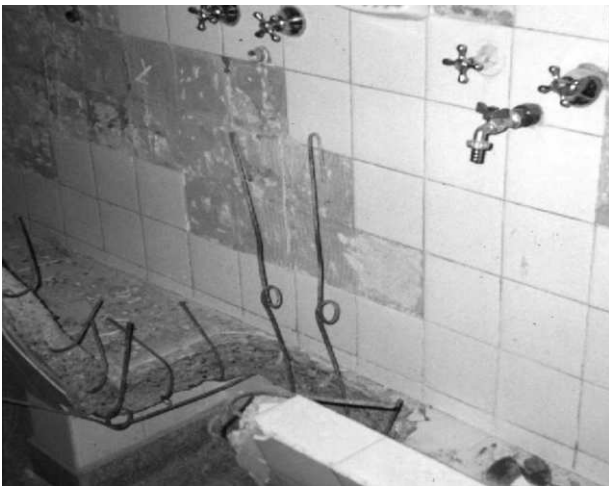
Figure 3. Explosion in sanitay linings.
