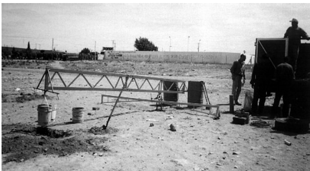
Fig. 7: Equipment general view.
