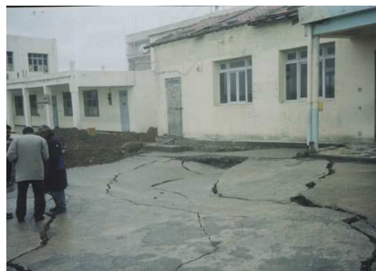
Figure 1. Sight on the course fissured
