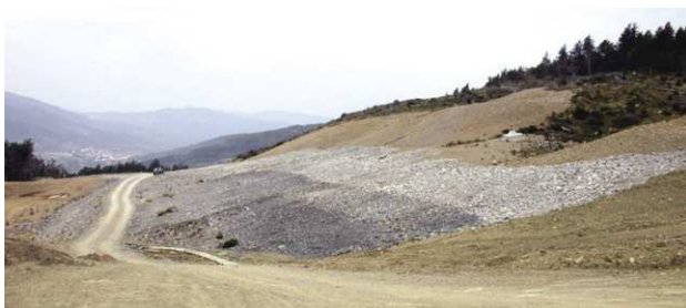
Figure 3. Toe of the landslide after backfilling
