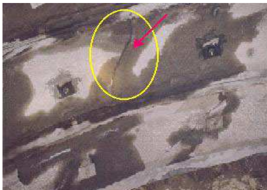
(a) Crack in the shotcrete near entrance
