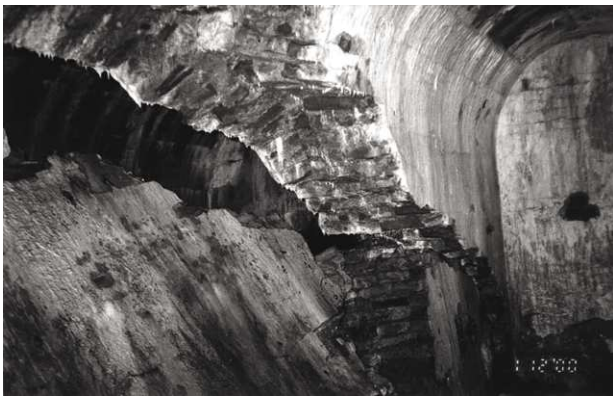
Figure 7. Dilapidated transverse cellar wall behind east section loggias (photographed in 2000)
