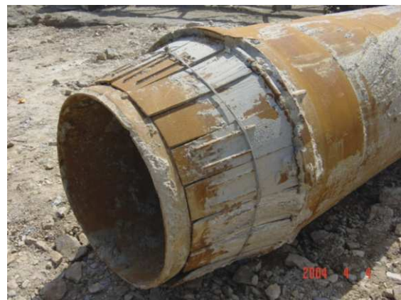
Fig. 5. End detail of temporary casing for cast-in-situ (PCC) pipe pile ( Liu et al. (2005) ).
