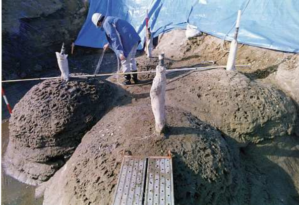
Figure 13. Photograph of soil improved by permeable grouting method, as exposed in an excavation at a field test site (Yamazaki et al.)
