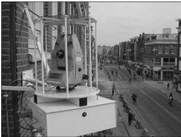
Figure 17. Automated total station in use for monitoring North-South line tunnel construction project in Amsterdam (Van der Poel et al, 2005)
