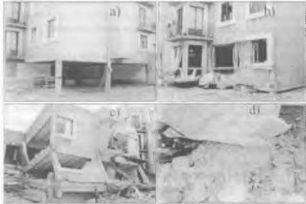
Figure 10. a) Story building with soft story in downtown Puebla, b) & c) Collapse of a building similar to a); and, d) close-up of the penetrated corner column in the ground for the building b).
