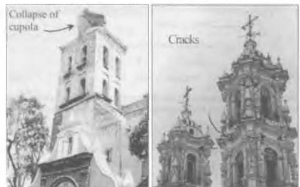
Figure 9. Cupola failure in San Agustin church, downtown Puebla, and extensive cracking at the bell towers of the Ocotlan Basilica, Tlaxcala.
