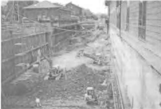
Figure 2. Overview of the excavation. To the right is Frederiksberg Centre, and to the left the Old Frederiksberg Station.
