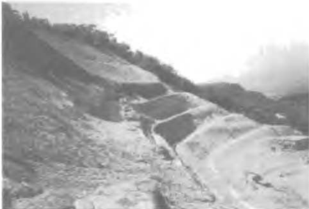
Figure 2. The 1995 slope failure.
