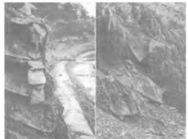
Figure 8. Decomposition and collapses of the wrapped face of the GRS slope.
