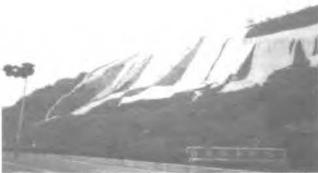
Figure 3. Front view of the failed GRS wall.
