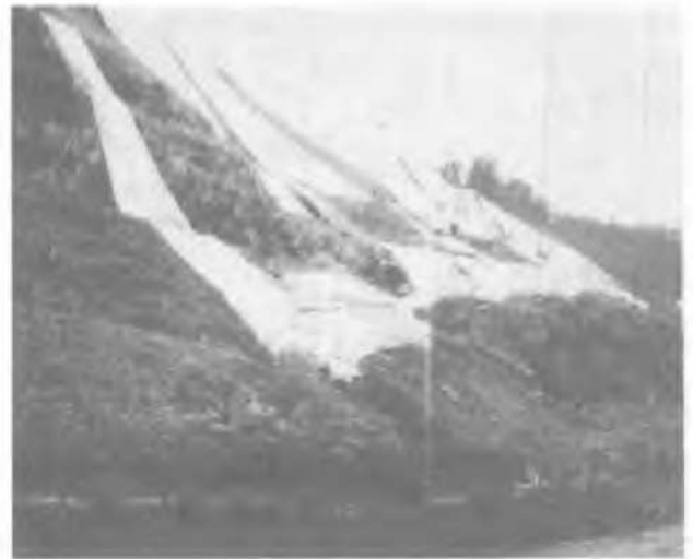
Figure 6. Side view of the failed GRS slope.
