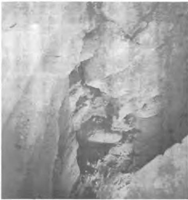
Fig. 7 Cracked stone foundation of a single pillar
