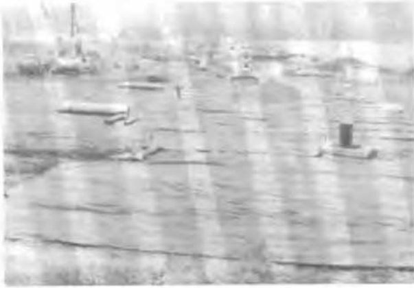
Figure 1: Geotextile placement on the grass and spreading of the gravel with a bulldozer.
