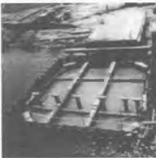
Fig. 4 Cofferdam just after the boiling failure occurred
