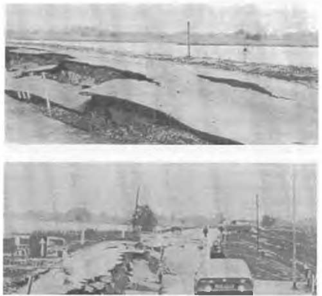
Figure 2. Uplift induced dike failure at Streefkerk, the Netherlands
