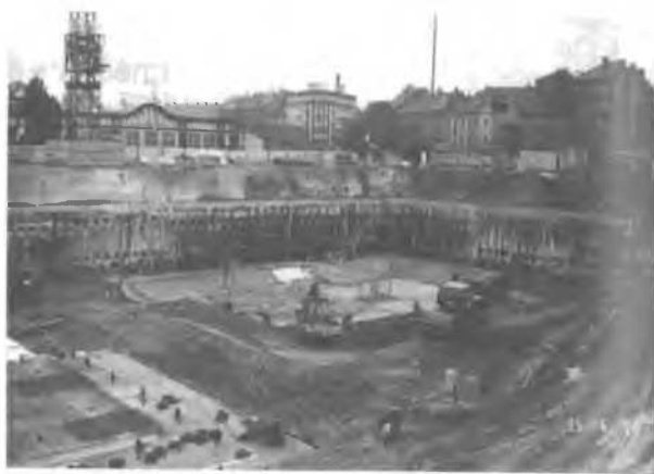
Figure 3. Excavation pit for General Credit Bank in Bratislava, safeguarded in the upper part with nails, in the lower part with prefabricated reinforced concrete walls.
