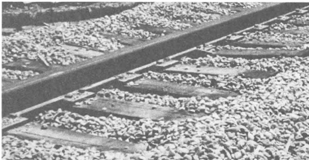
Figure 6. Ties split on tie centre line below rail.
