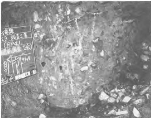
Fig.52 Crack development at the pile head, Pier 211 (Hanshin Highway Authority, 1996)
