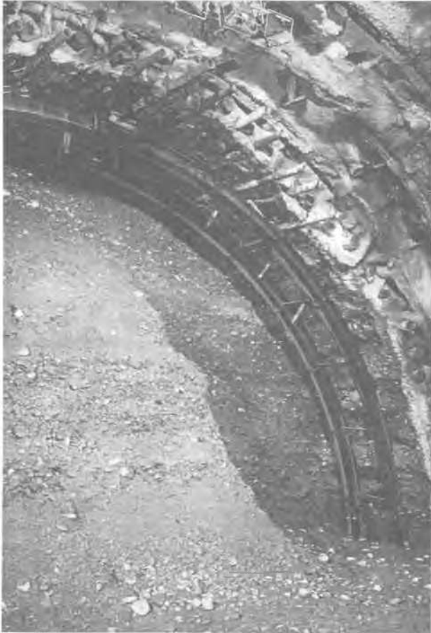
Fig. 6 - Photograph of the ground conditions at the face in the underground tunnel. Details are shown of the jet-grouting columns and steel pipes as used according to ground treatment and pre-support system 1.
