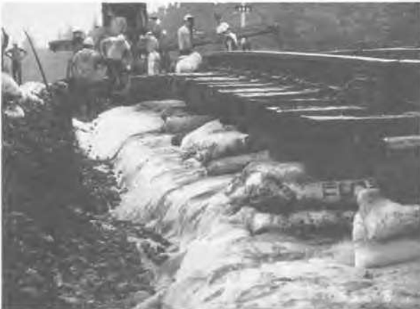
Figure 11. The installation crew has drapped geotextile into cut trench to allow the geotextile to facilitate drainage.
