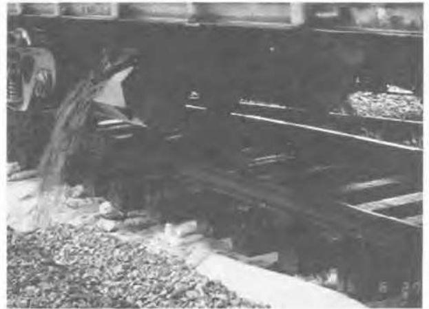
Figure 12. Trench should be filled first to result in tensioning. Ballast filled side trenches promote drainage as long as outlet pipes are installed.
