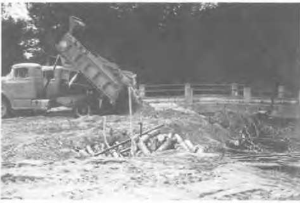
Figure 14. Note in-place berm in foreground with tree logging reinforcement ready for placement within the central load bearing area.
