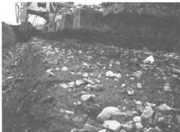
Figure 9. Stone particles left after undercutting will eventually pierce a lightweight geotextile.
