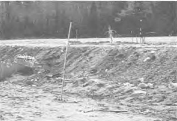
Figure 16. Large differential settlements occur at small changes in loading.
