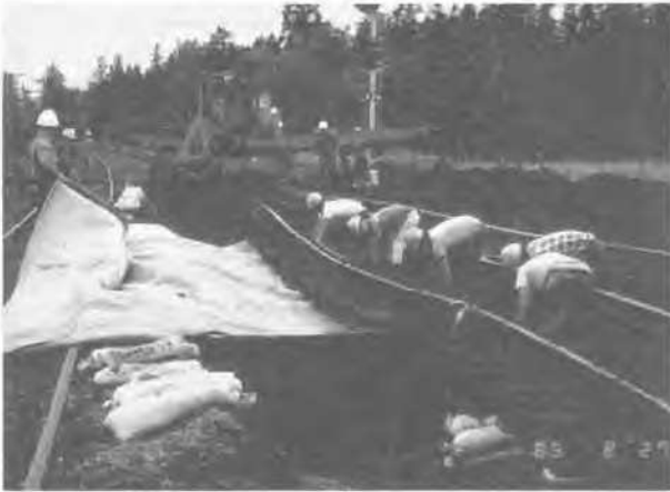
Figure 10. Geotextile installation below tracks. At all times, geotextile should be handled and installed with care.
