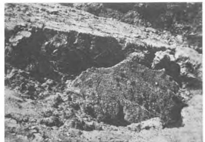
Fig.8 Collapsed sinkhole on downstream side of dam.
