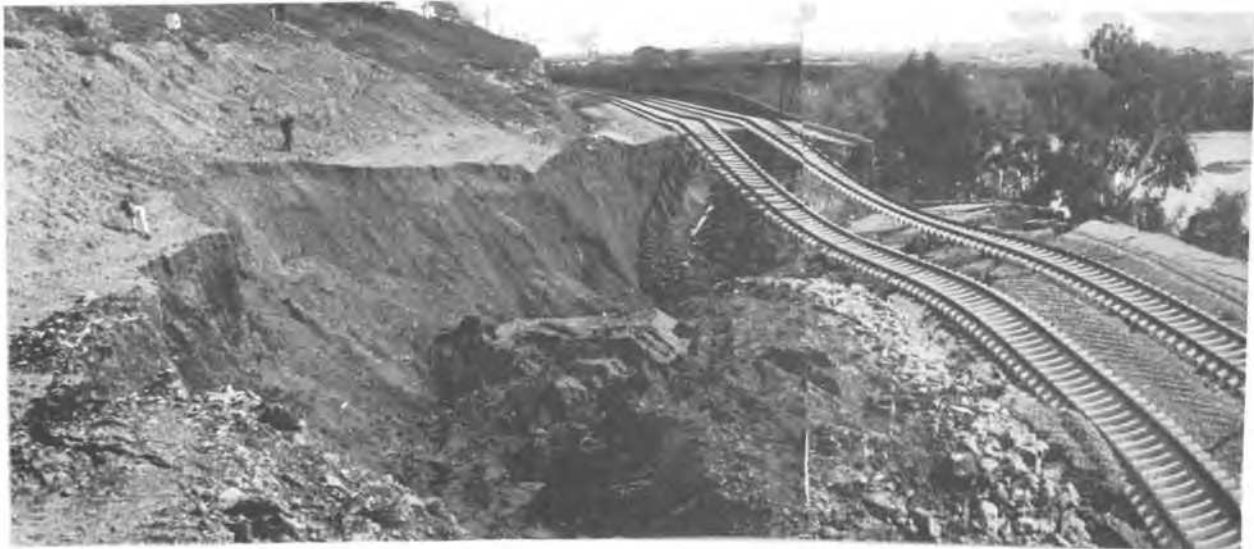
Fig 2.-General view of the landslide
