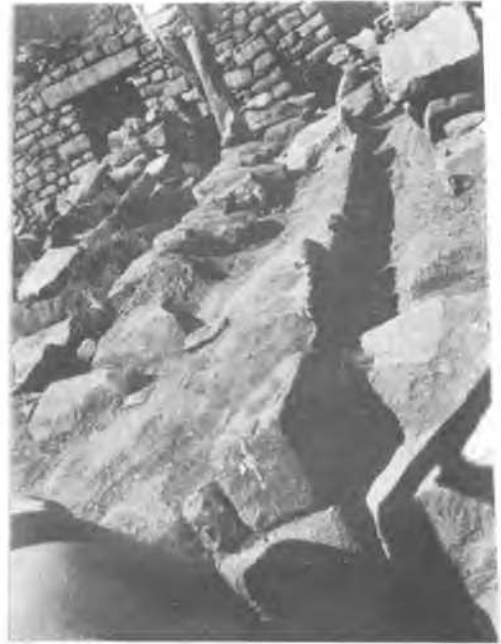
Fig. 2 Stepped foundations in stone for the absorption of seismic movements, Cuzco, Perú
