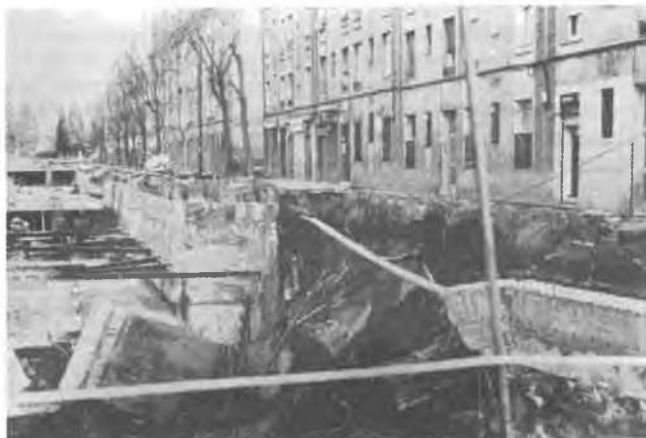
Fig. 1. Overturning of a diaphragm wall by yielding of the struts. Observe the displaced foundation pit (marked by an arrow).
