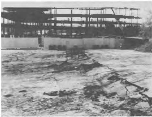
FIGURE 5 SUBSIDENCE VISABLE AFTER PILE CUT-OFF
