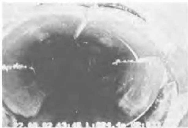
Figure 1: Broken stoneware pipe
