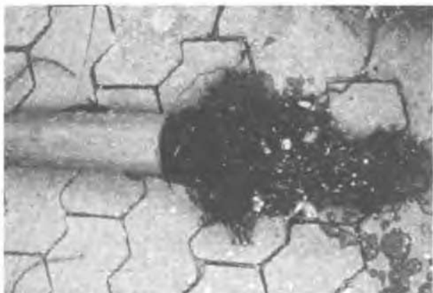
Figure 4: Ingrowing of roots in a drain pipe
