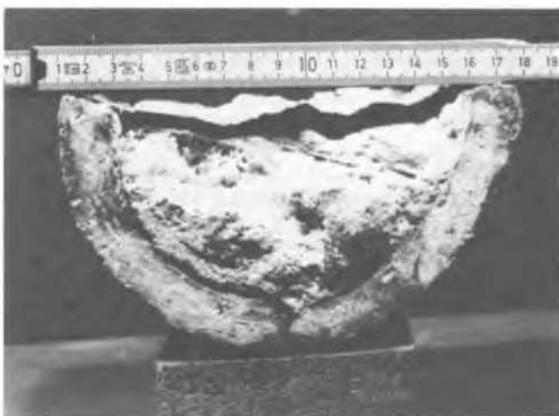
Figure 5: Removed drain pipe with sinter deposits
