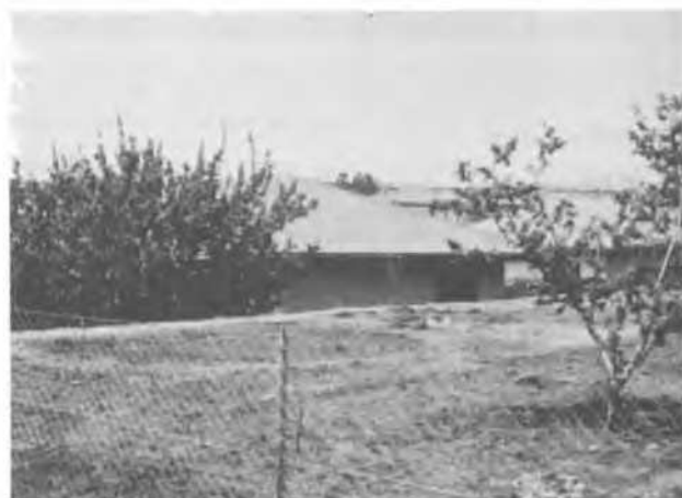
FIG. 6: ACTIVE WATER TABLE - UNCRACKED HOUSE WITHIN DOLINE AT LUPIN PLACE CARLETONVILLE - 1963
