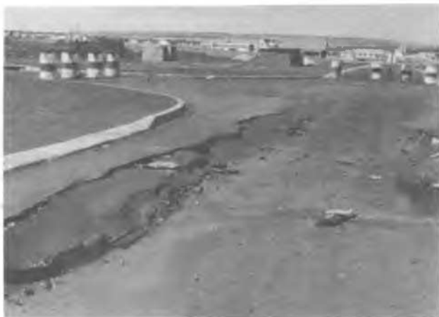
FIG. 4: STATIC WATER TABLE - DAMAGE TO ROAD DUE TO COMPACTION SUBSIDENCE AT NEW DEVELOPMENT
