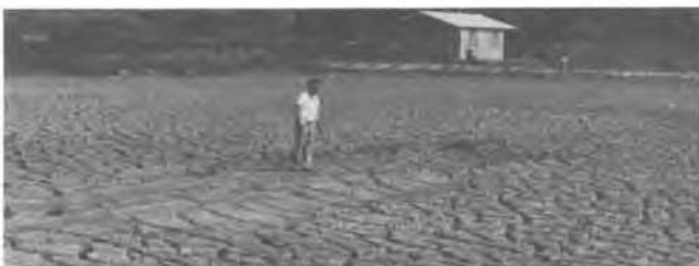
Fig. 5 - Differential settlements in correspondence and in the vicinity of a ridge, basin 6. Crack spacing in the ridge is larger than in the adjacent zone.
