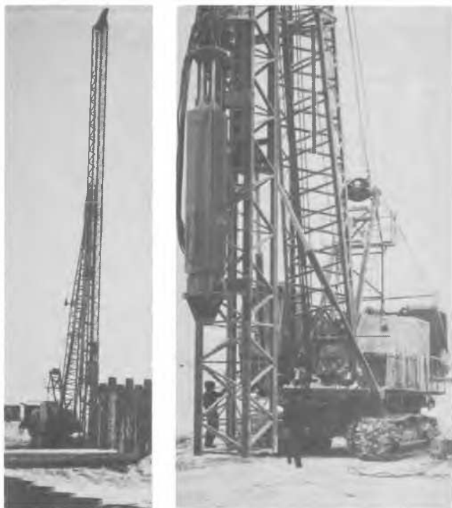
Fig. 3a) Driving of the pipe pile wall and 3b) the 80 kN hydraulic drop hammer, Junttan.
