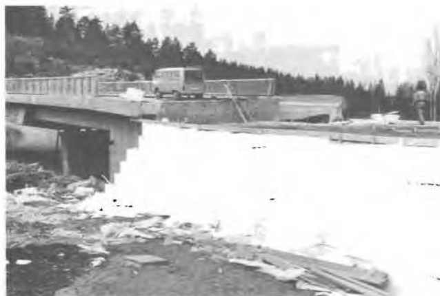
Fig. 1: A 4,2 m high fill of expanded polystyrene in Oslo. The use of polystyrene blocks reduced the bridge by one span. (Photo: Ulf Winther)
