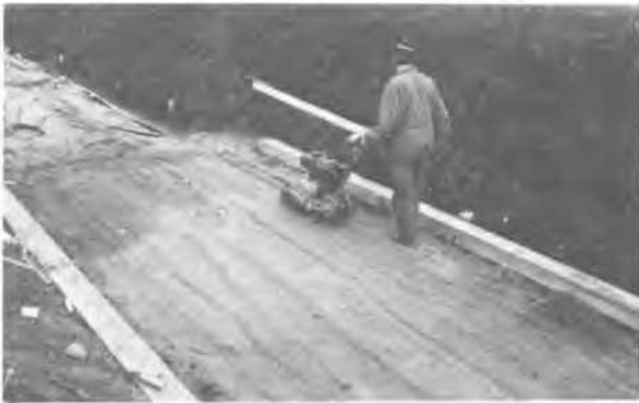
Fig. 3 Compaction of the test blanket. The soil, bentonite and water are previously mixed in a concrete mixer.
