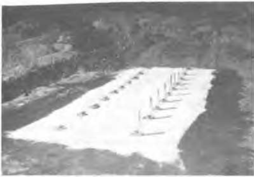
Fig. 6. - Two rows of extensometers for measuring tensile strain in the embankment surface.
