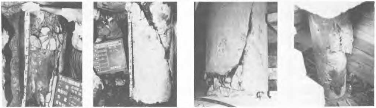
a) Case 1 b) Case 1 c) Case 3 d) Case 4 Fig. 1 Typical Examples of Damaged Piles
