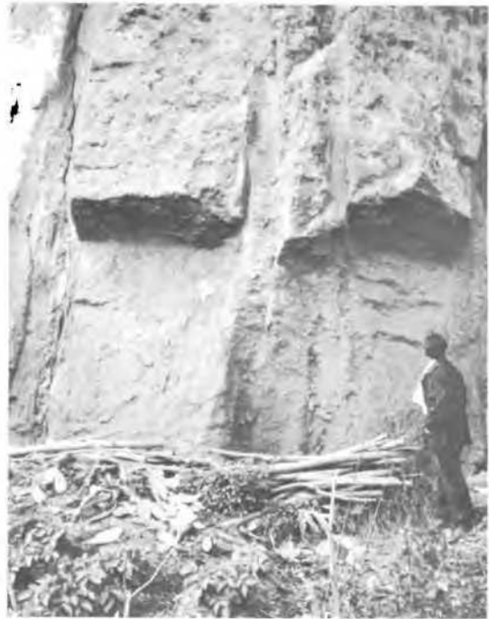
Fig. 10 - Portions of overhanging rock
