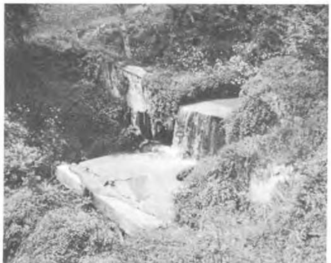
Fig. 11 - Broken and displaced check-dam; water infiltrating into the clay formation
