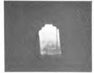
Fig.3 Plumb Line showing inclination of 7th Story.
