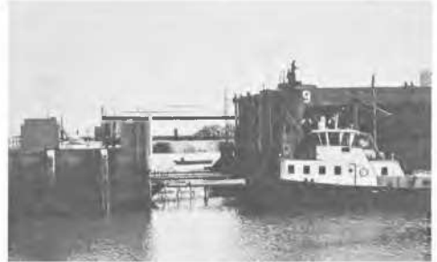
Figure 4 Between the test caisson on the left and the reaction caisson on the right the hydraulic jacks to provide the cyclic loading forces are clearly visible
