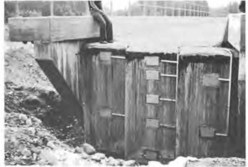
Fig. 4. Instrumentation of the northern buffer plate with Glötzl-type earth pressure cells.
