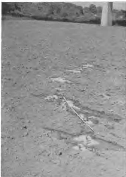
Fig 2. A crack from which sand and water flowed out
