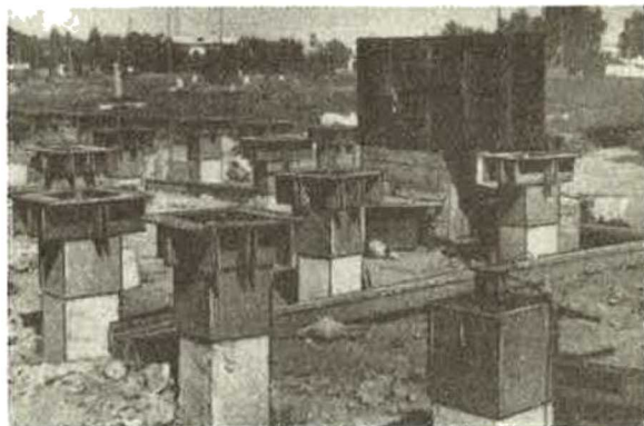
Fig. 1. Part of installation of stringed dynamometers upon the heads of piles of the experimental houses in the Karaganda coal basin.
