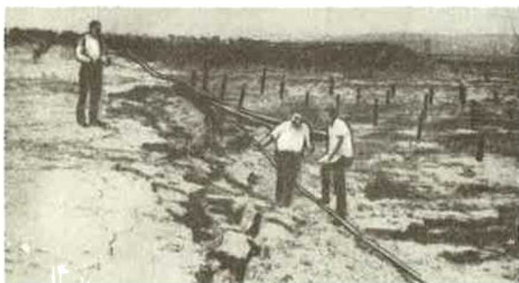
Fig.3. To the right-the soil surface, collapsed to the depth of 1.4 m after compactation; to the left-the lot before the compactation.
