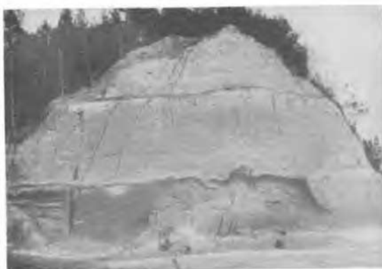
FIG. 10. AN EXAMPLE OF BRITTLE FAILURE IN CUT-OFF SLOPE
