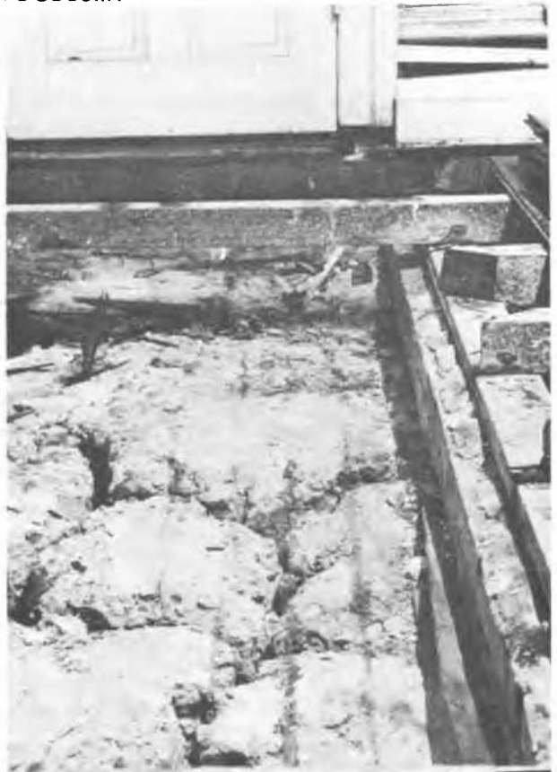
Figure 2. Crack pattern at surface beneath timber floor in Adelaide Steamship Building, Adelaide, South Australia (see suction profile in Figure 1).
